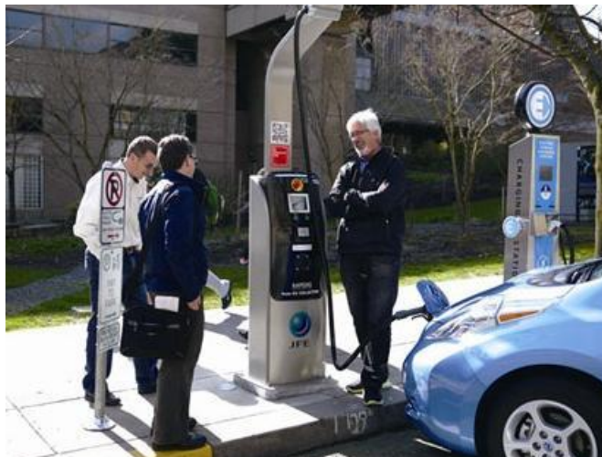
Figure 11: RAPIDAS / Kanematsu 208 volt Battery Backed Fast Charger on Portland's "Electric Avenue" 15
